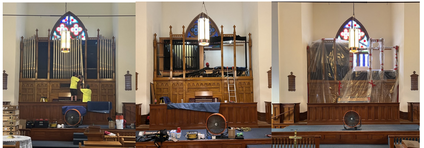
On September 11, 2023, the historic tracker organ in the sanctuary, installed in 1905, was partially disassembled—all exposed pipes removed—and the entire case covered in plastic to protect it from falling debris and dust.
