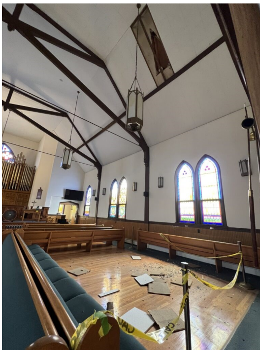
On July 1, 2023, a large section of ceiling tile failed leaving a large hole in the sanctuary ceiling.
