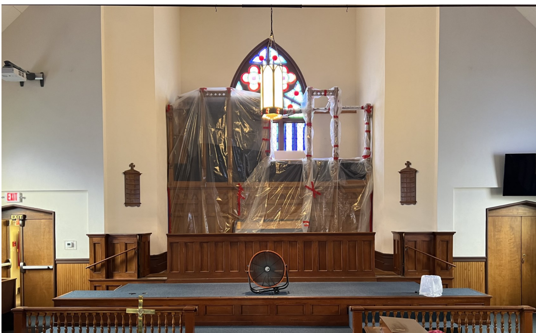
On September 11, 2023, the historic tracker organ in the sanctuary, installed in 1905, was partially disassembled—all exposed pipes removed—and the entire case covered in plastic to protect it from falling debris and dust.
